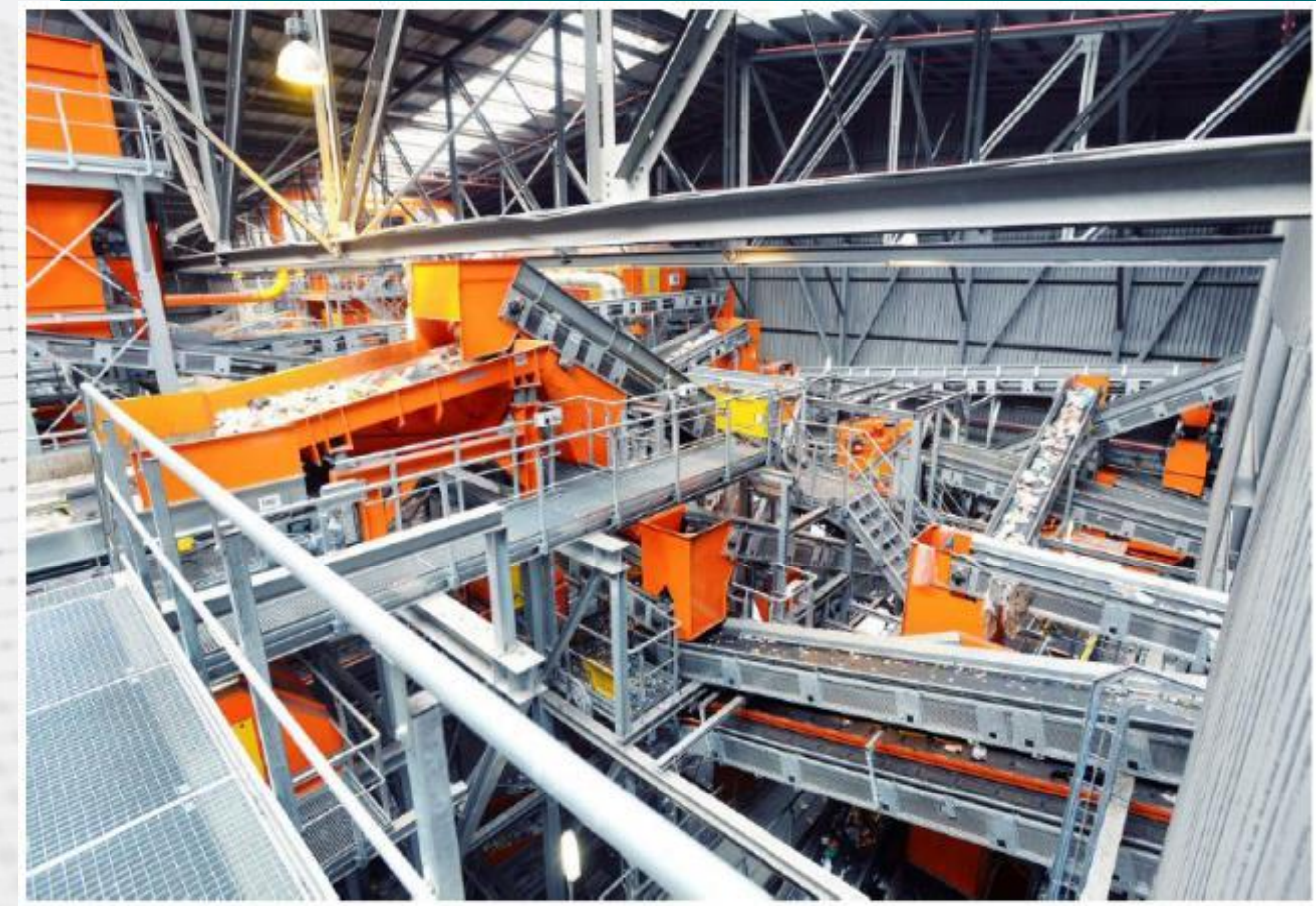
Sorting plant for lightweight packaging Quelle: PREVENT Waste Alliance, 2020, EPR-Toolbox
